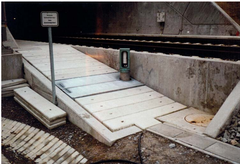
Fig. 3 Measuring weir in the cable terminal shaft of the Freudenstein Tunnel
